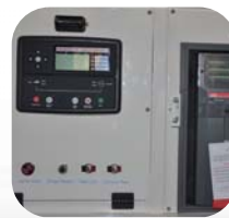
Control Panel & MCB
